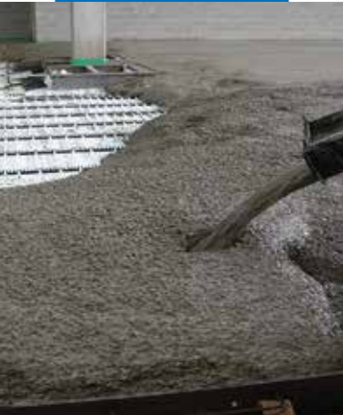
Pouring concrete with the addition of Mapefibre NS12 to counter plastic shrinkage
