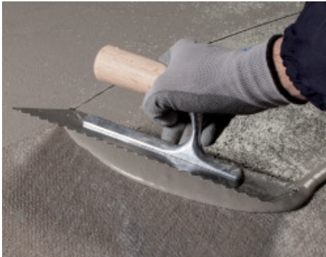
Application of the second coat of Mapelastic Turbo over the first coat reinforced with Mapetex Sel N
