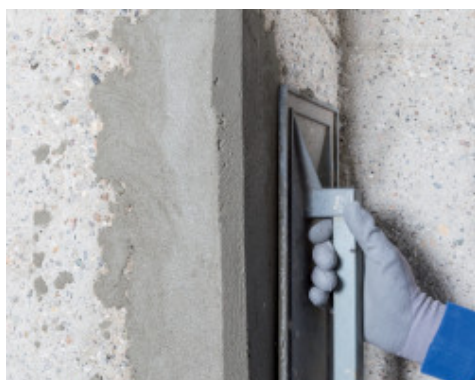
Floating the surface of Planitop Smooth & Repair R4 to create a smooth finish
